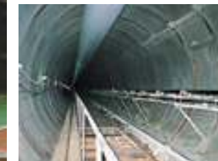
Ring beam supports
